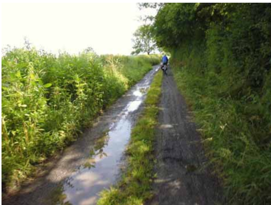
The road north from Lendales Farm is in need to refurbishment.
